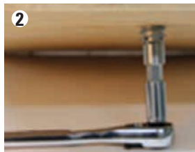
2 Level- Place countertop on cabinet & adjust level from underside with ratchet & shim driver
