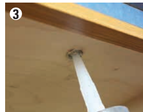
3 Glue- Apply adhesive through center hole of Twist Shim to permanently lock counter in place
